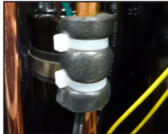
Figure 6: Thermistor attached to the refrigerant line.
